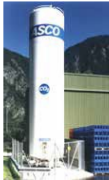
Vertical CO 2 storage tank
